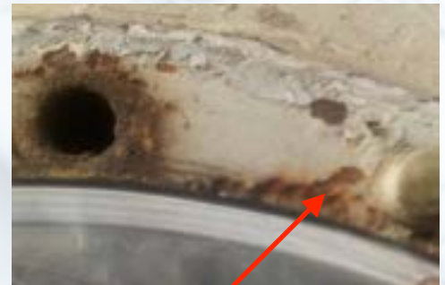
Droplet/Pitting Corrosion (Refrigerant Tank)
