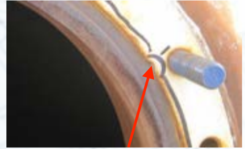
Broad Surface Corrosion (HF Acid Tank)
