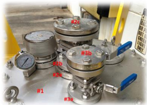
Figure 1: Front View of Tank Connections
