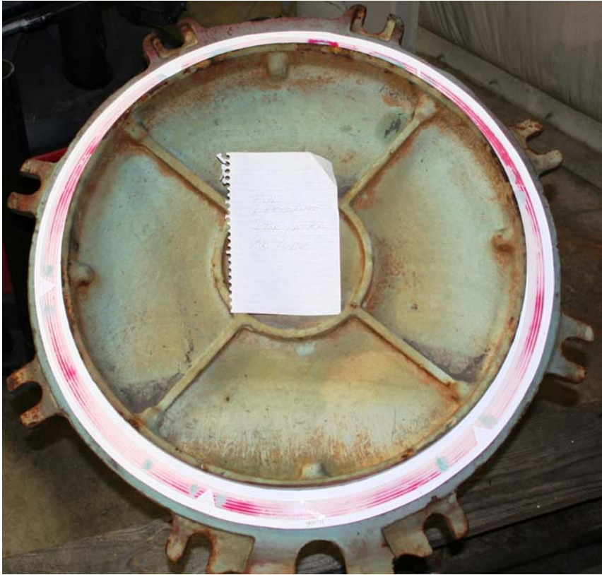
Unlubricated Eyebolts Non-Uniform, Lower Overall Gasket Stress
